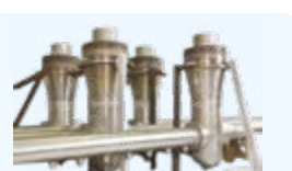
Hot collectors/ headers
